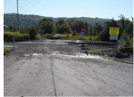
2 55 th Street – Passive warning device only
